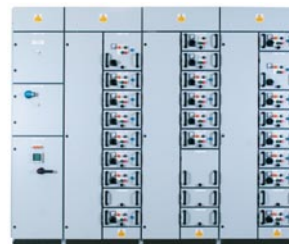
MOTOR CONTROL CENTRES
